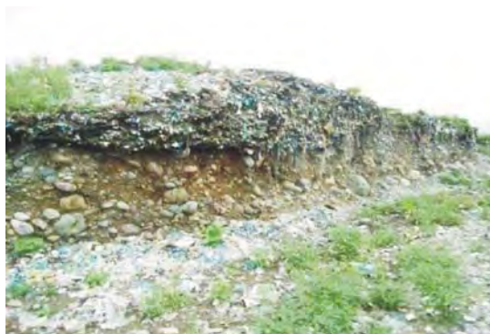
Figure 7. Waste being washed away by flood
